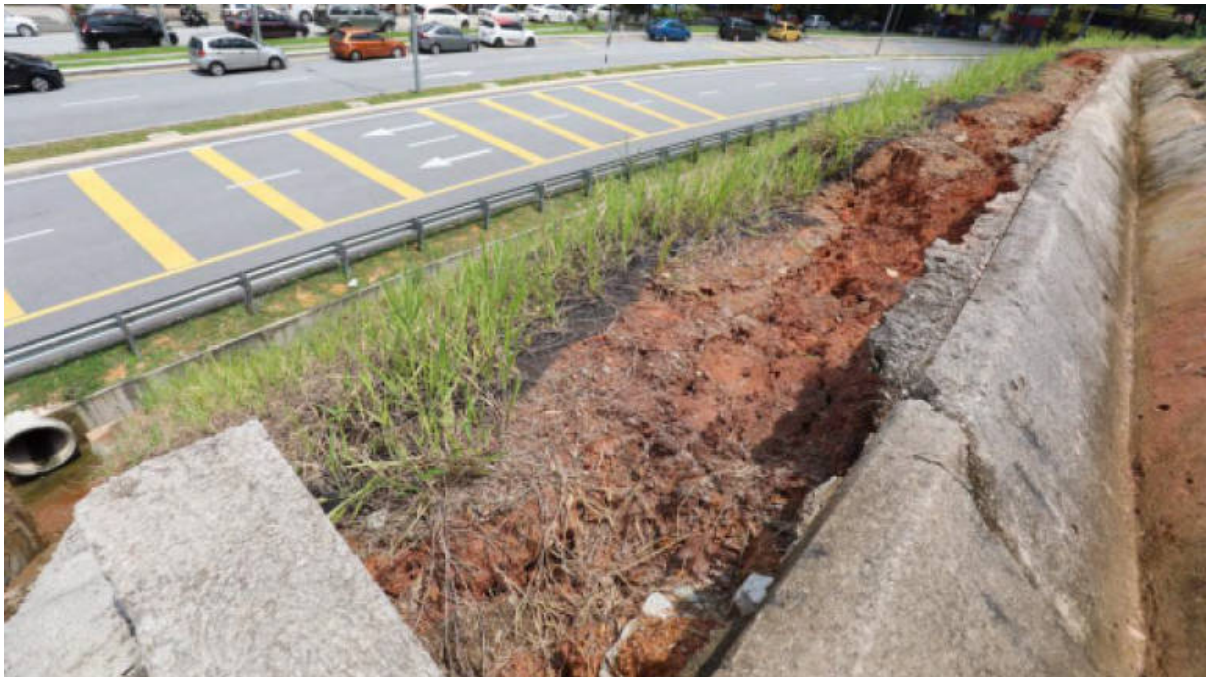
The cliff along Jalan 11 / 55C, Puncak Setiawangsa, Bukit Setiawangsa appears to have fissures measuring half-a-metre, in this photo taken on, May 12, 2017. — Sunpix by Amirul Syafiq Mohd Din
